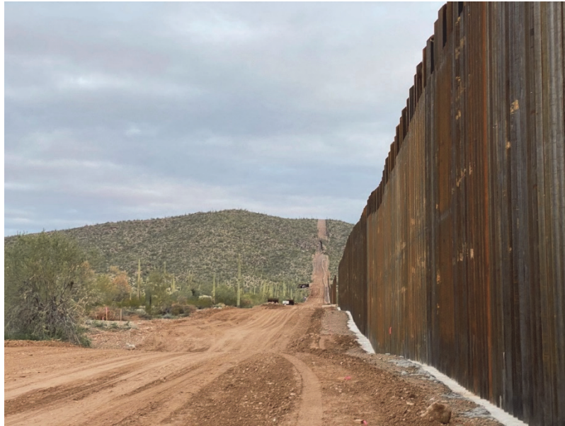
After construction at Organ Pipe Cactus National Monument (same location). Photo: Laiken Jordahl
